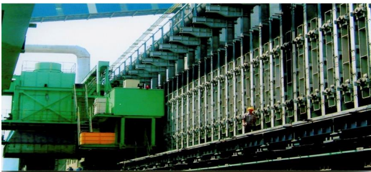
Coke oven from view from Pusher side (Fig-1)
