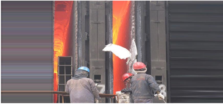
Blanketing of ovens for repair ovens using ceramic fibre blanket refractory wool Temp: 1000 degree centigrade (Fig-3)
