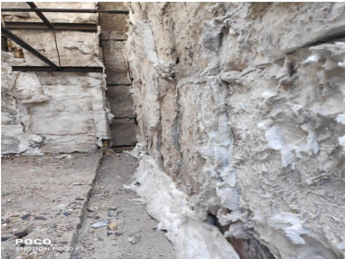
Heating wall created for work: In side heating wall temperature 800 to 1000 degree centigrade (Fig-4) ambient temperature about 50-60 deg centigrade
